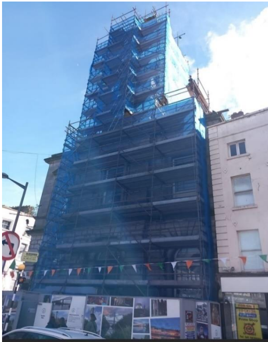
Photo shows the extensive temporary works necessary to access the roof at Tholsel
