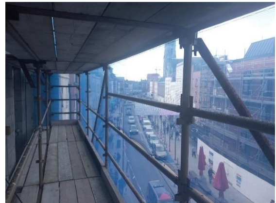
Photo shows one of several temporary works platforms necessary to access the roof at Tholsel
