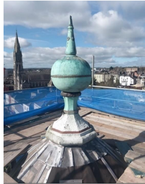
Photo shows lead work at the roof of Tholsel which will be replaced and the Copper Ball.
