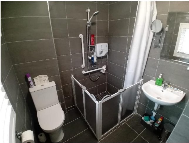
Bathroom Adaptation completed in March in Ardee, assisted with a Housing Adaptation Grant
