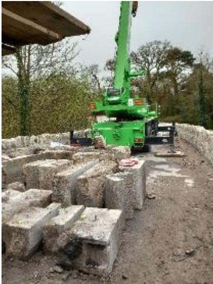
Dismantled abutment Stone (labelled for reinstallation), also rebuilt stone walls from Southside of River Boyne
