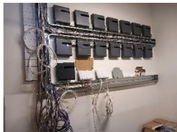
Comms cabling Block n
