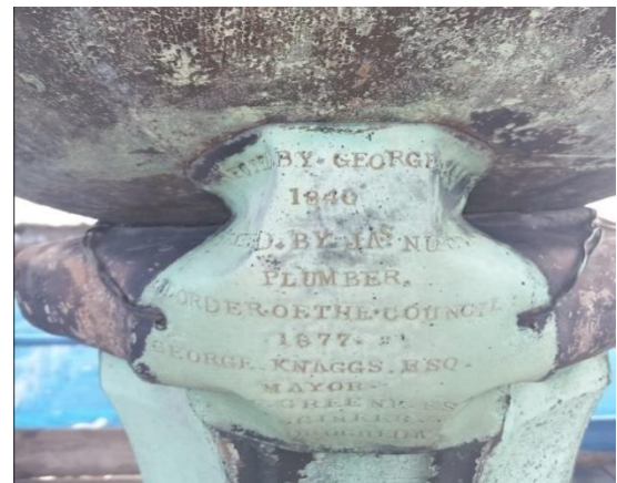
Photo shows an inscription at the roof of the Tholsel with dates of 1840 and 1877
