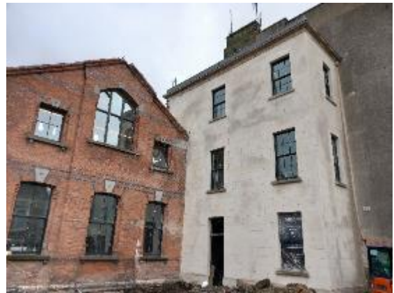
Block C (Brick) and East Front Elevation Block E (Plastered) with both new and refurbished windows. Parapet Lead to Roof Block E.
