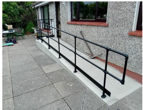
Ramp installed in May in Dundalk part-funded by a Housing Adaptation Grant.
