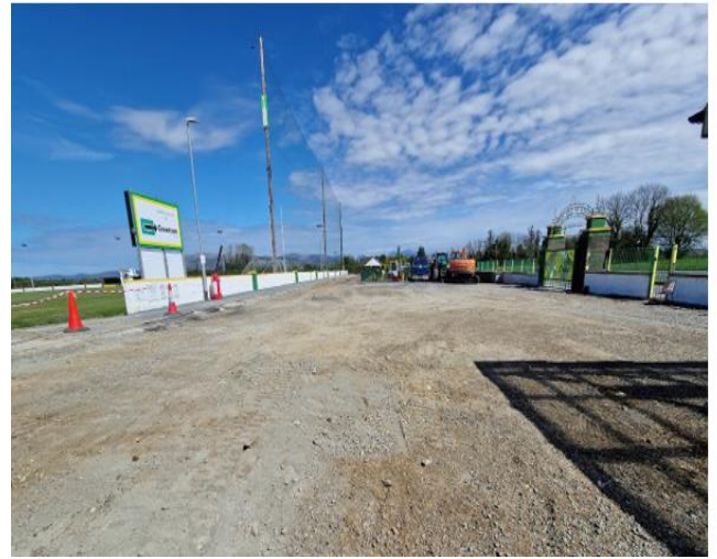
Cooley Kickhams GFC Carpark before upgrade
