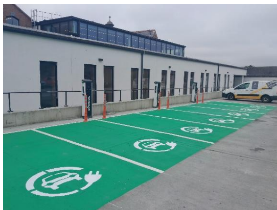
EV Charging Infrastructure installed
