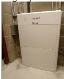
New 10kWh battery pack installed in the Council's Animal Pound at Whiterath
