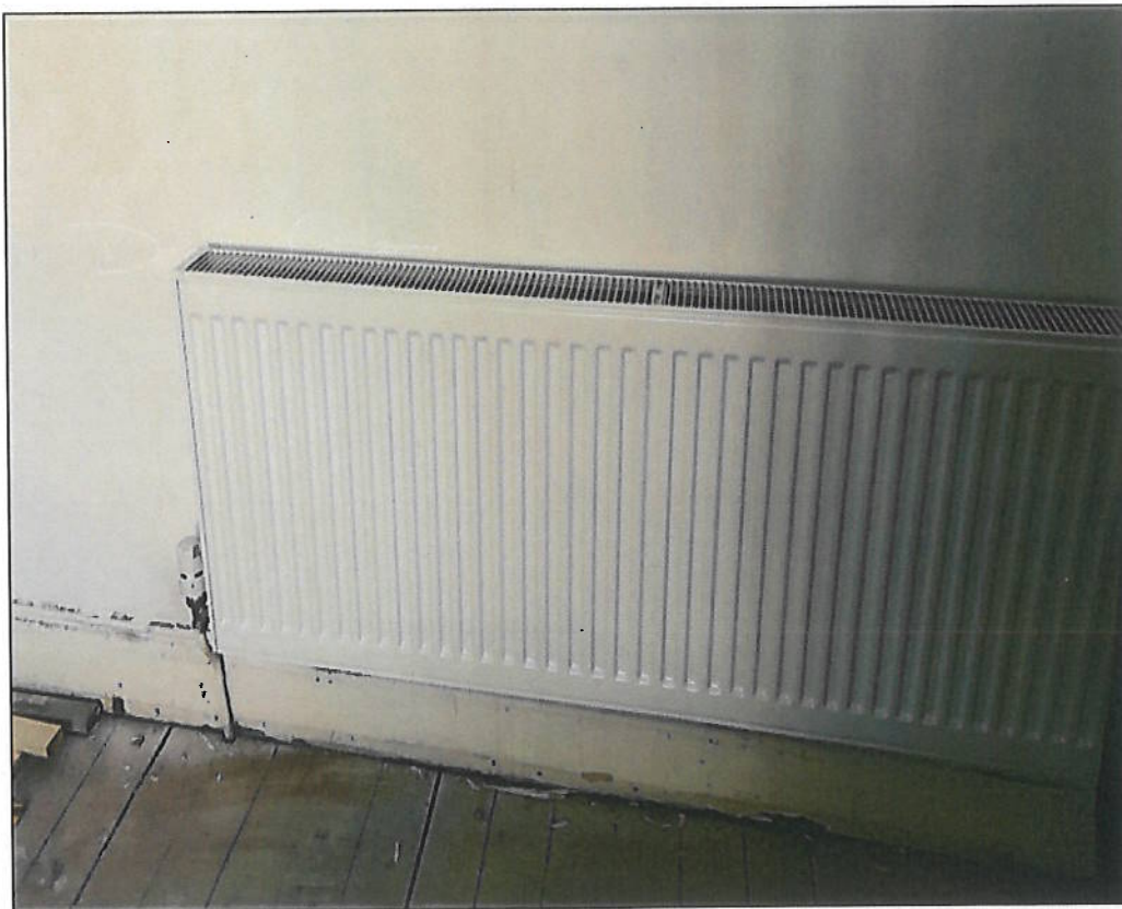
New radiators to replace existing ones – they still have retained existing radiators and are available for inspection (see below)
