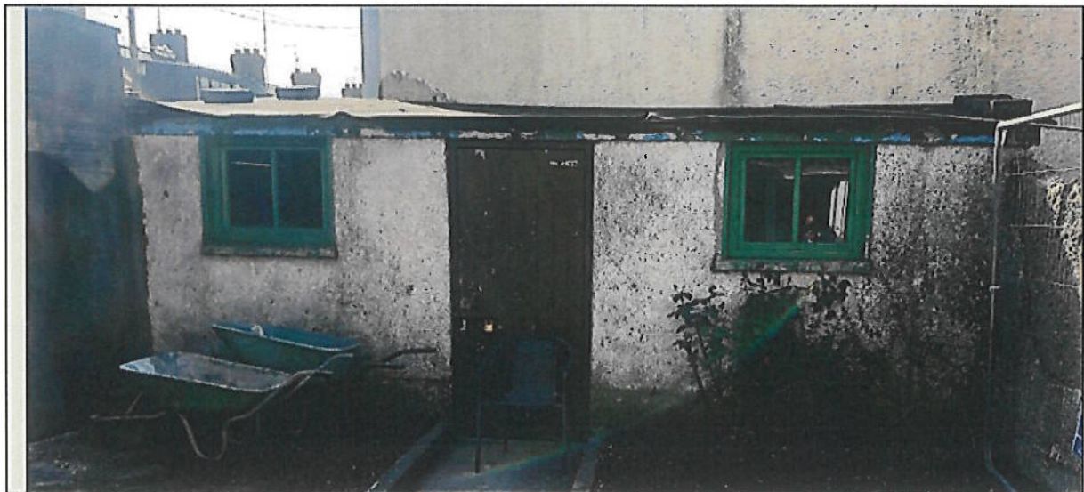
Figure showing outbuilding in yard where clients want to repair – roof needs re-felting, repairs to window & doors + repainted
