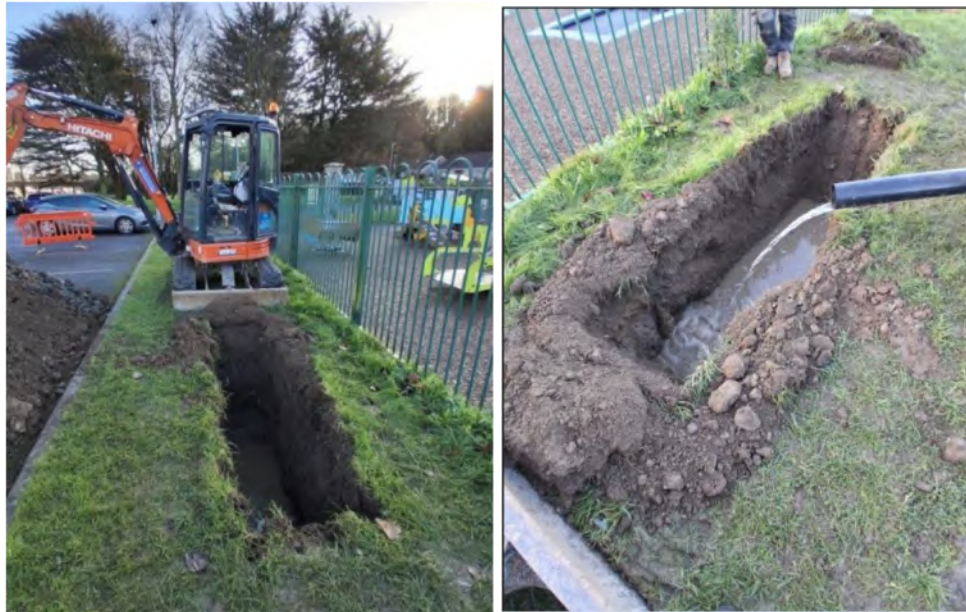
Plate 16. Ground photographs of trialpitting and BRE365 testing carried out to the north of the playground carpark to determine the suitability for a SuDS system
