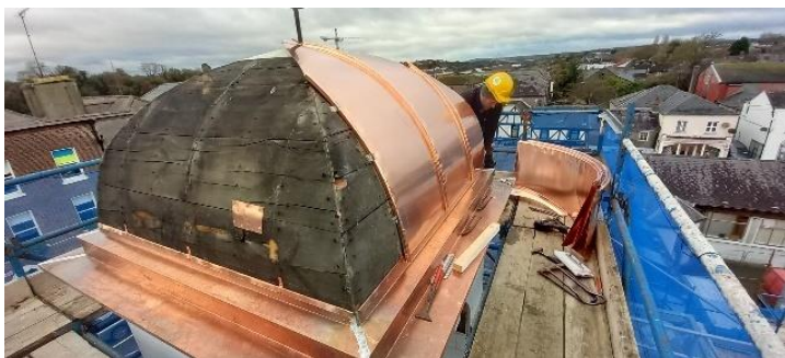
Progress to renovate the cupola at the Council Office, Fair Street, Drogheda.
