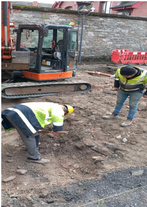
Construction works On the Learning Pod for the Varcities Project at the Open Space at the County Library
