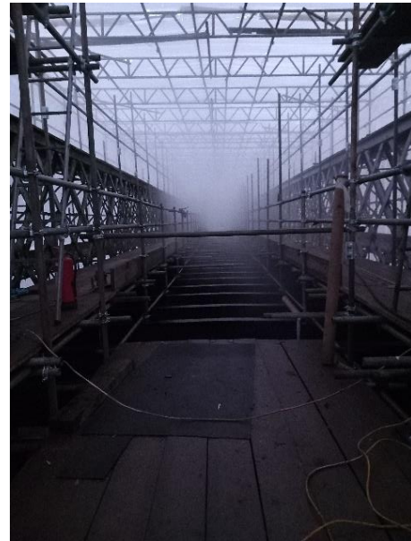
Mist rising from power washing of steel prior to shotblasting inside encapsulation.
