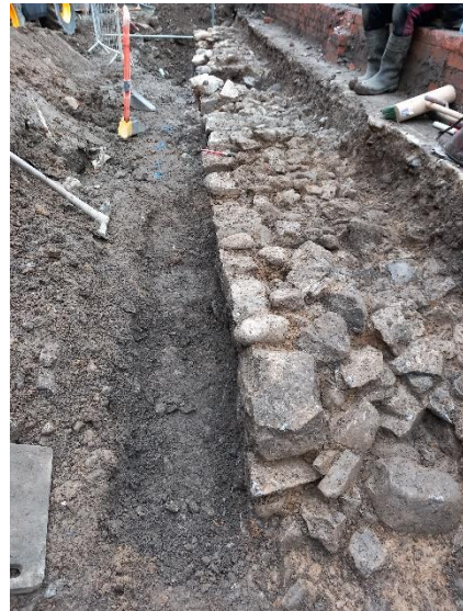
Block C (South Side) -Archaeological Dig -Old Town Wall unearthed, surveyed, protected and backfilled to allow progression of RC planter Walls
