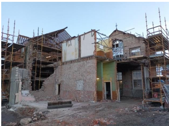
Subsided North and West Elevations of East Wing of Block C removed
