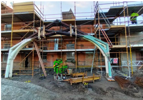
Removed Trusses from demolished section of Block C, to be reinstated within the new build.
