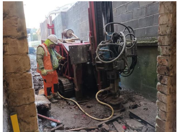
Mini Piling Rig driving piles to Underpin adjacent boundary walls with no foundations
