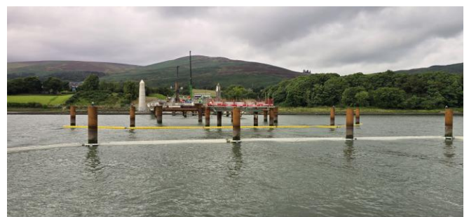
Floating Fender Collision system installed.
