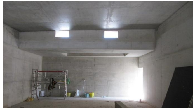
Internal view of plant room – North side.
