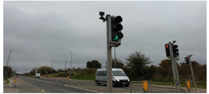
New Traffic Light Radar installed at Monasterboice pedestrian crossing giving added protection to pedestrians - lights will not turn red when close convoy of vehicles approaching
