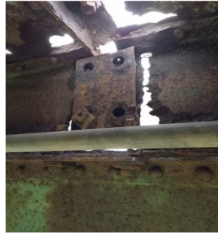
Steel members and splices plates on underside of bridge to be upgraded
