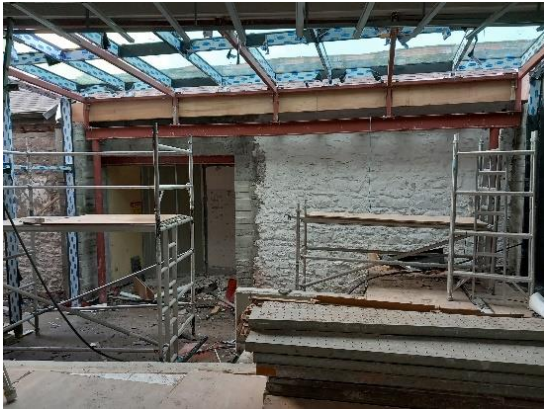
Block N New Link Building : Breakout area linking New Build to existing Francis Johnson Building
