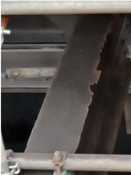
Close up of corroded Main Horizontal Steel Member
