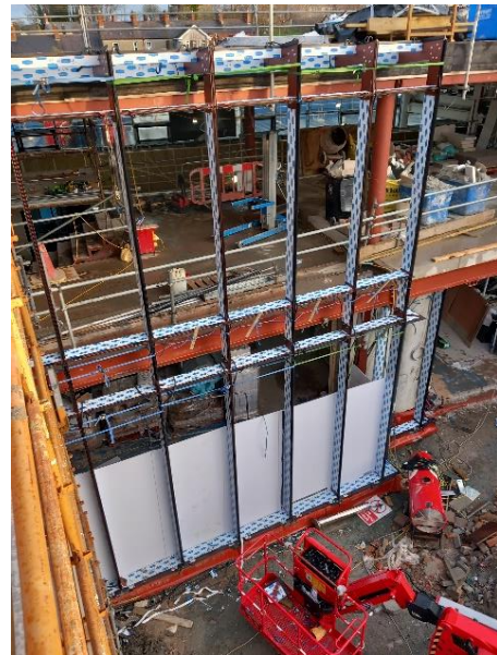
Block N New Link Building : Entrance Copper Façade Support Frame Structure installation
