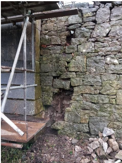
Damaged Stone southside of Bridge.
