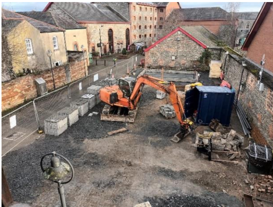
Construction Work in Progress for Varcities Project at County Library and Museum
