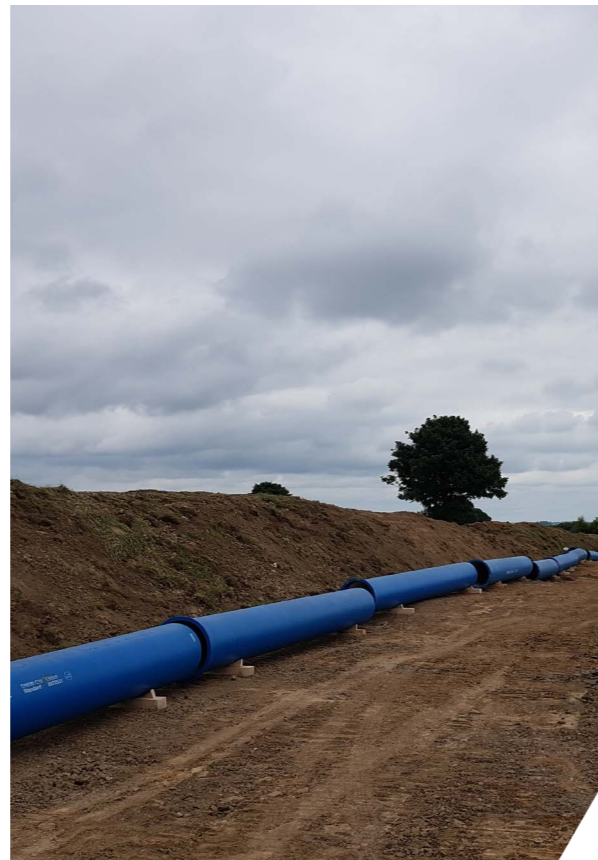
Staleen Water Treatment Plant.
