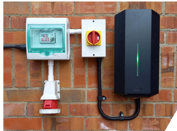
EV Charging Point for staff.
