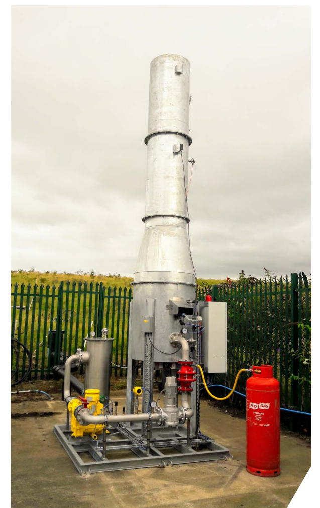
New low-cal gas flare installed at Drogheda Landfill.
