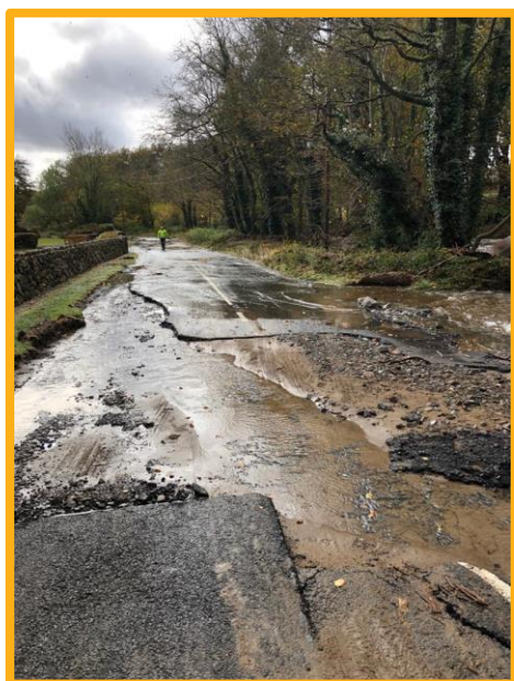
Figure 3.14. Road damage as a result of extreme rain, Louth 2023.
