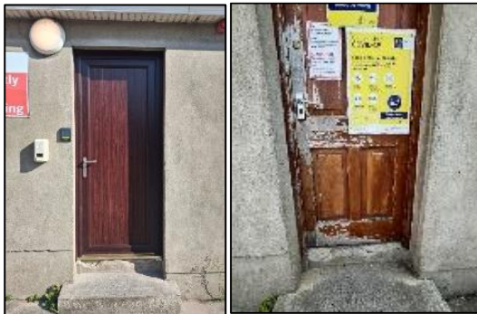
Photos: Improvements to external door at the Machinery Yard at Fair Street, Drogheda.
