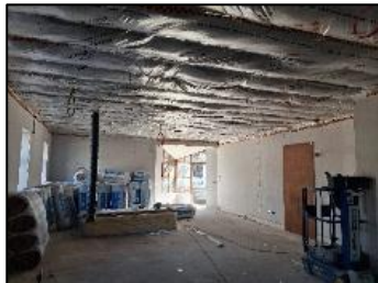
Photos: Work in Progress at the Cornmarket Building at Fair Street, Drogheda
