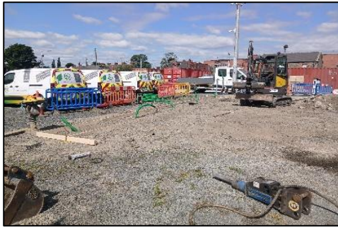
Photo: Civils works in progress for New EV Charging Facilities at Dundalk Machinery Yard
