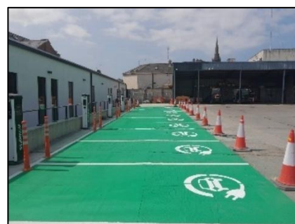
Photos: New EV Charging Facilities at Drogheda's Machinery Yard
