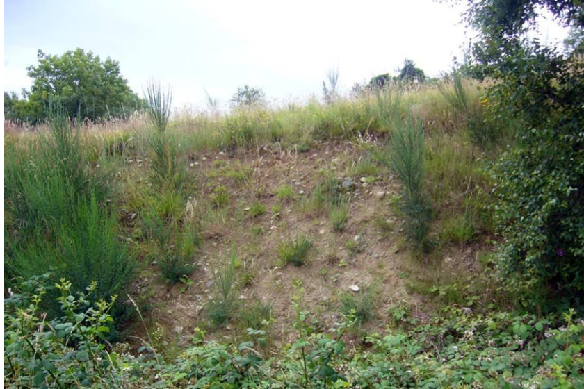
Plate 10.12 Infill material in area of former cutting for Greenore to Newry Railway.
