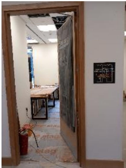
Block N Secure Meeting Room (Glazed Table to Ceiling to be installed)
