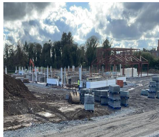
Insulation to Rising Blockwork in Place. External Brickwork Plinth to SNU Commenced
