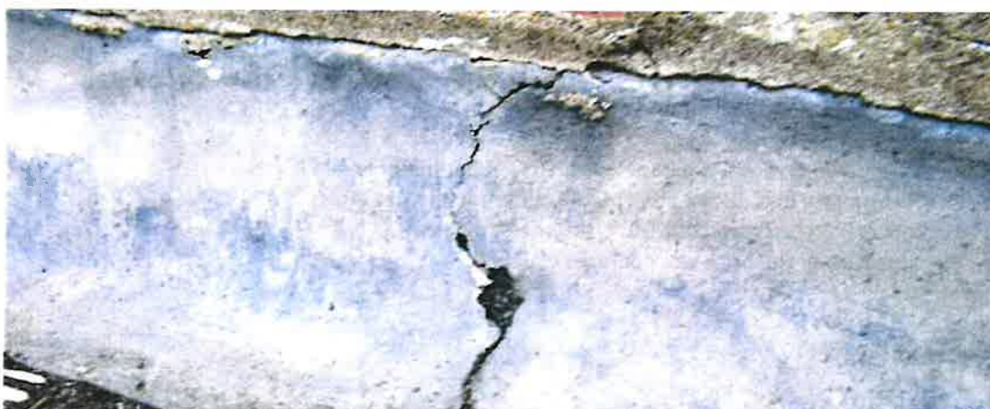
Damage to lead cavity trays.
