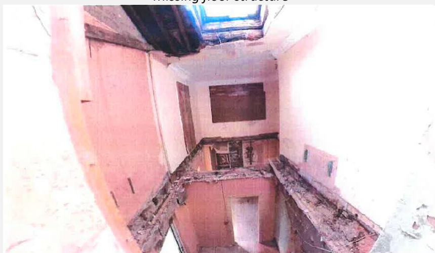
Missing floor structure
