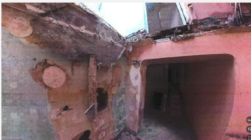
Missing floor structure
