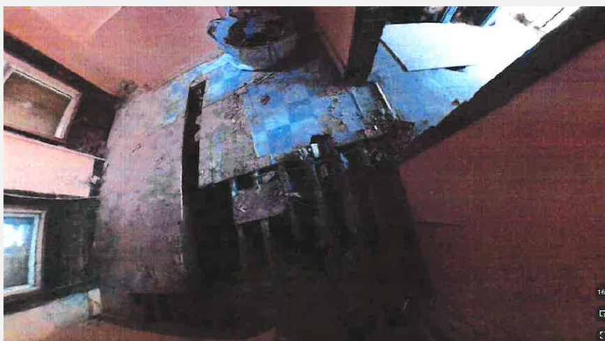
Badly rotted floor structure
