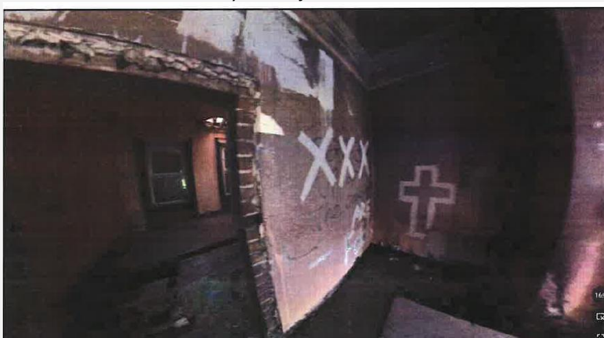
Fire damage and graffiti
