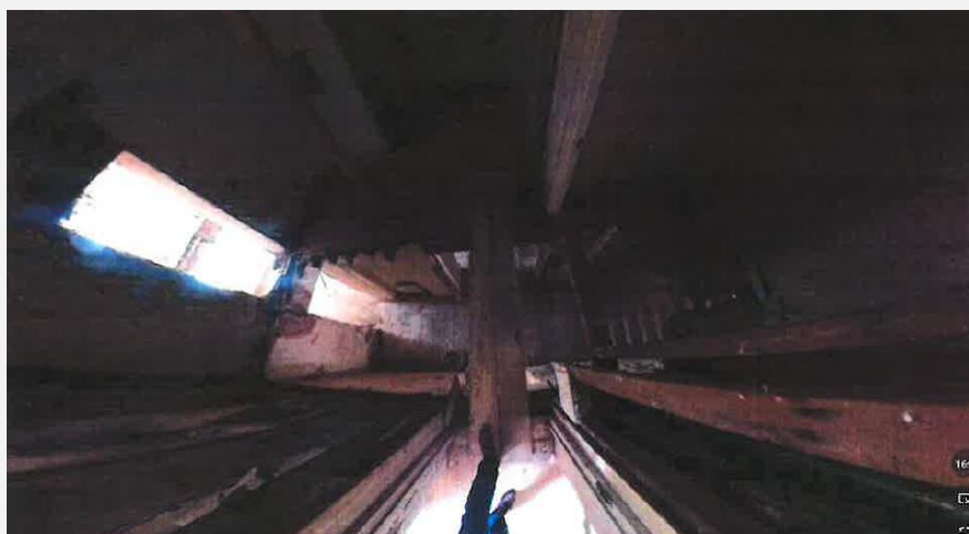
Badly rotted floor structure
