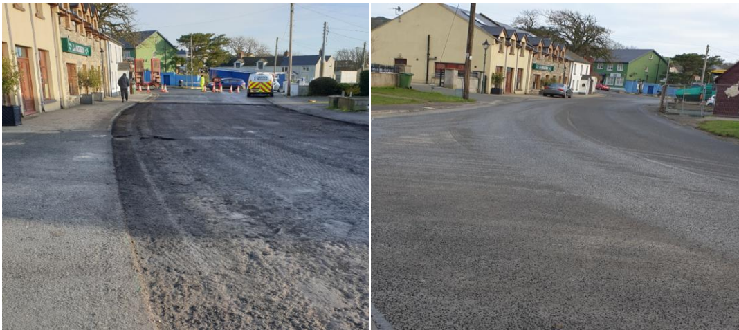
Clogherhead Junction with Callstown (R166 with the LS-6283-0) Photos show Resurfacing Works underway and completed works
