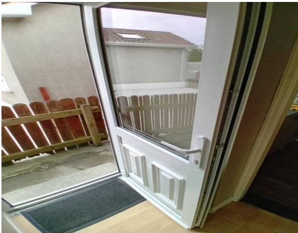
New door fitted in June in Dundalk, part-funded with a Housing for Older Persons Grant
