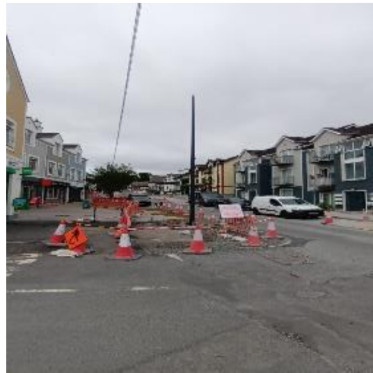
New Public Lighting on Station Road
