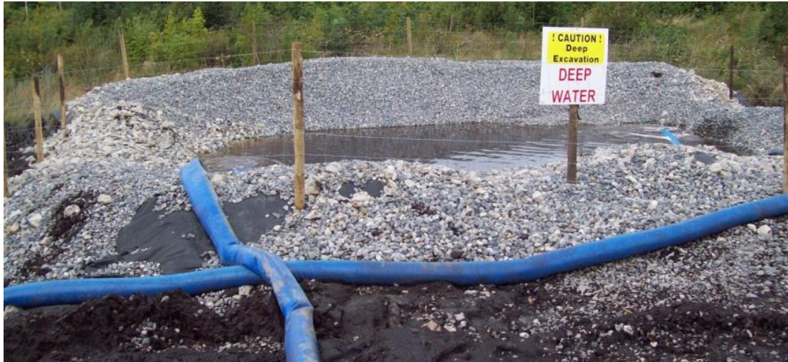
Figure 5 Typical temporary settlement pond/lagoon
