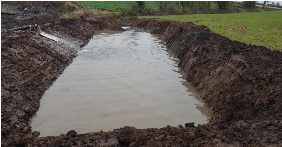
Figure 6 Typical temporary settlement pond/lagoon
