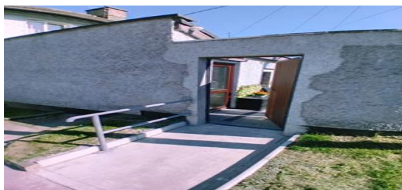
Ramp completed in May in Drogheda, with funding provided with a HAG
