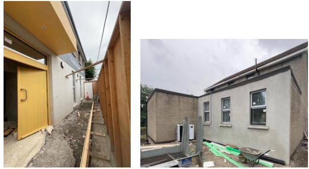
Photos show the improvements in progress to the front of the building and the repaired external wall at the rear.
