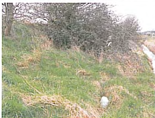
Photo 54 – chainage 1975 No more berm from back face toe to ditch
