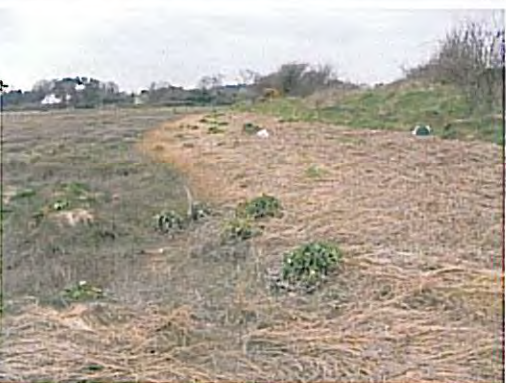
Photo 53 – chainage 1975 Rock toe and berm disappearing
