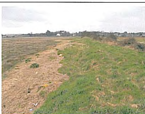
Photo 44 – chainage 1680 Change in shape of the embankment
