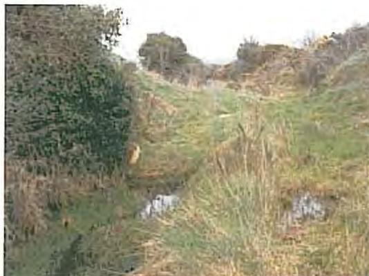
Blockage of drainage ditch
