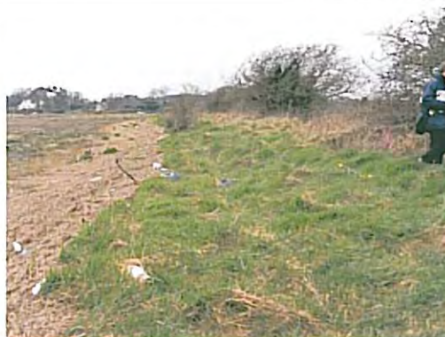
Photo 52 – chainage 1937 Berm and front face growing together
