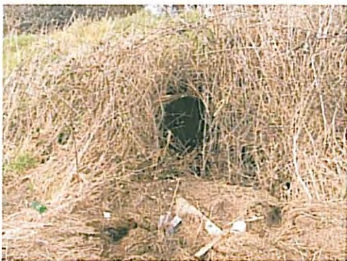
Photo 11 – chainage 478 Animal hole through the embankment
