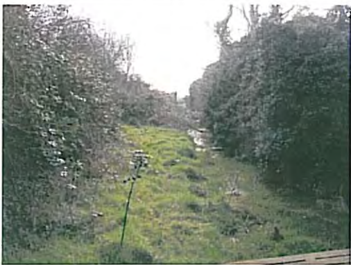
Photo 71 – chainage 0653 Ditch with heavy vegetation
