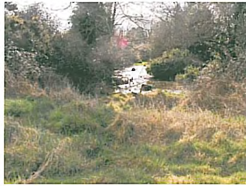
Photo 70 – chainage 0572 Blockage of the ditch
