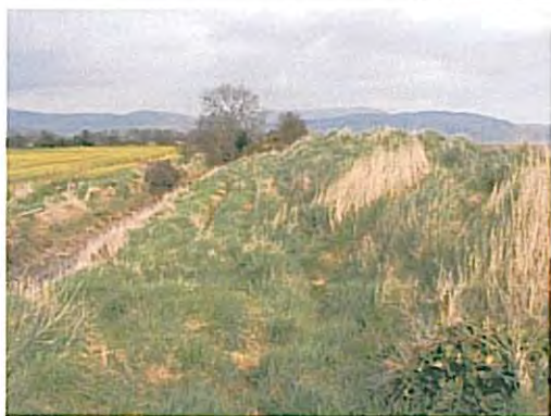
Photo 34 – chainage 1275 Back of embankment at outfalls
