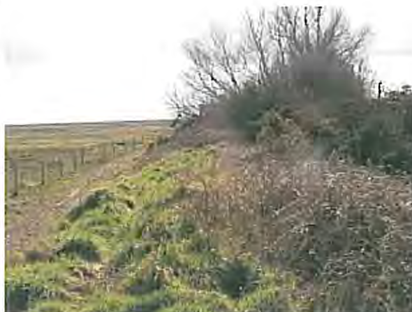
Figure 3-1 Heavy vegetation on the embankment
