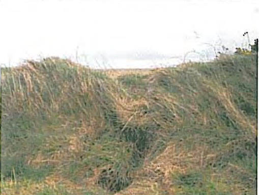
Photo 27 – chainage 932 Weak spot in the embankment back
