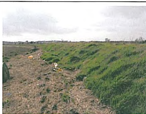
Photo 40 – chainage 1402 Front face dip and much debris
