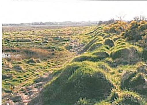
Photo 28 – chainage 1058 Vulnerable section of embankment
