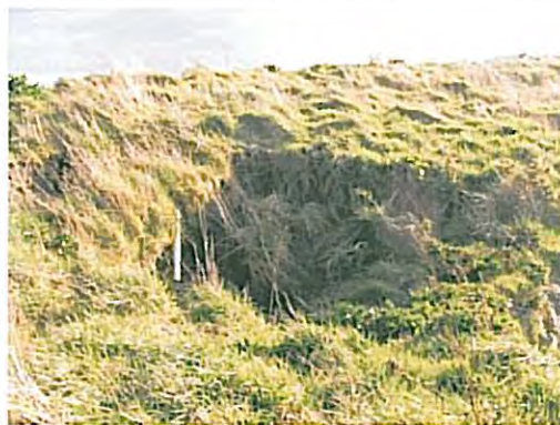
Photo 22 Hole in the back face of the embankment
