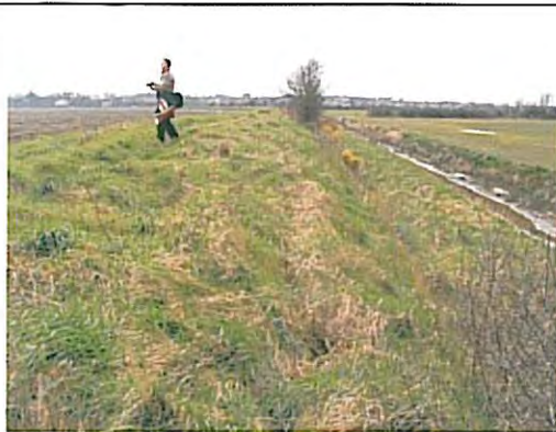
Photo 39 – chainage 1327 Slipped look back face
