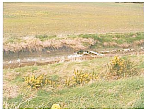
Photo 76 – chainage 1380 Form of cloth in ditch
