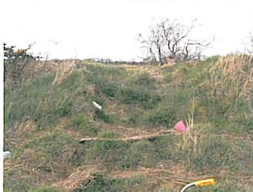
Photo 26 – chainage 932 Weak spot in the embankment front
