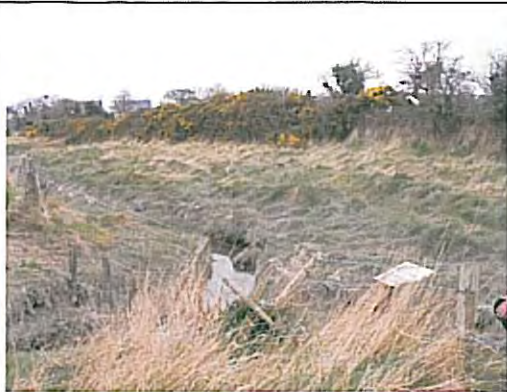
Photo 63 – chainage 2302 Embankment around corner
