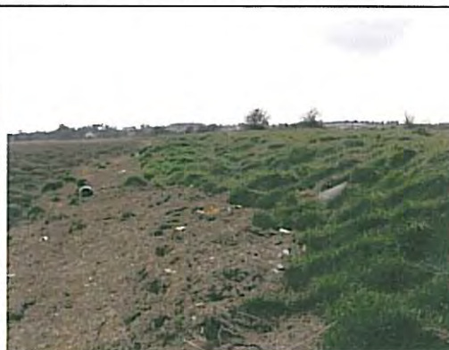
Photo 42 – chainage 1500 Front face of embankment changes
