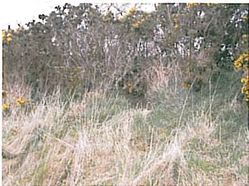
Photo 65 – chainage 2408 Gap in embankment
