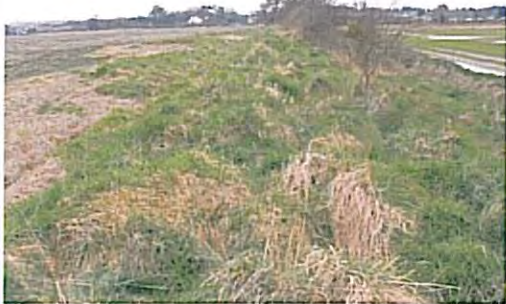
Photo 49 – chainage 1717 Uneven crest bad condition and grass berm in distance
