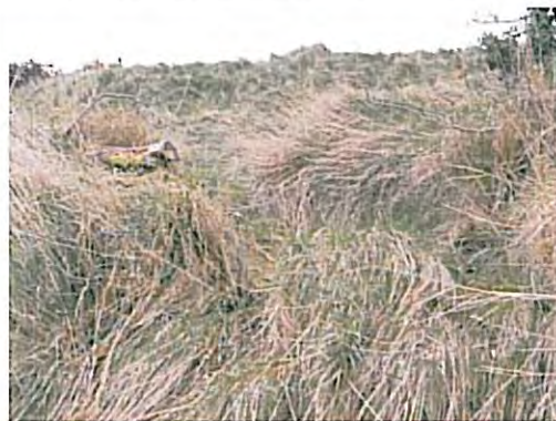
Photo 66 – chainage 2475 Weak spot on embankment
