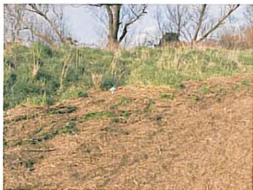
Photo 12 – chainage 218 Location of possible breach
