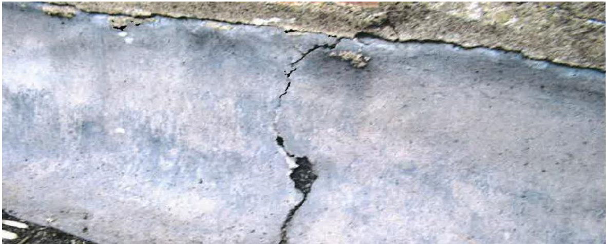
Damage to lead cavity trays.
