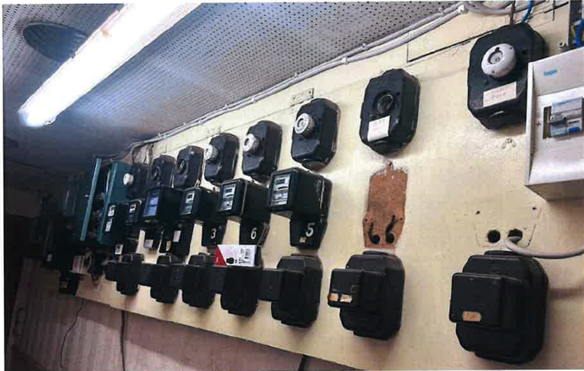
Figure 4.0 Image showing the electric meters for each apartment
