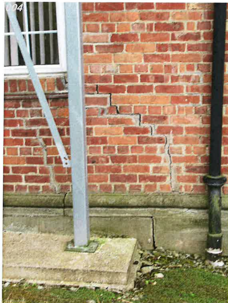
Structural cracking to external walls along rear of building
