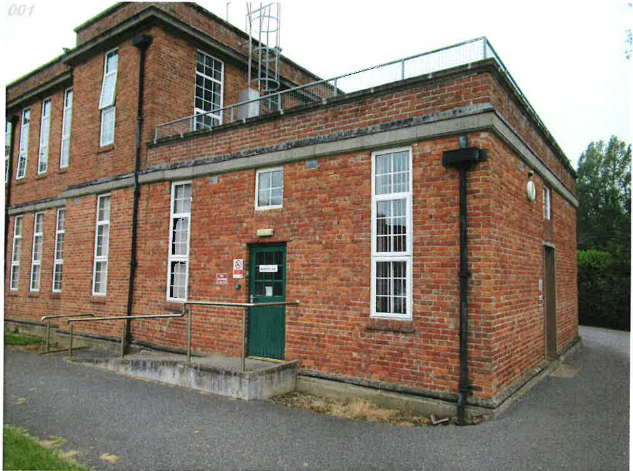
General view of single storey building wing in need of structural repair
