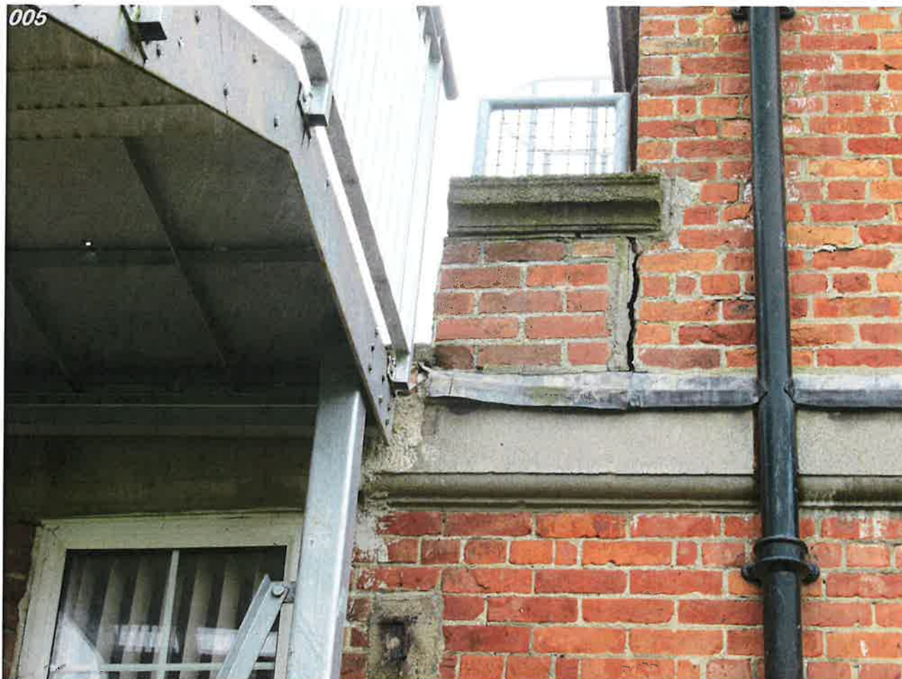
Structural cracking to rear of building
