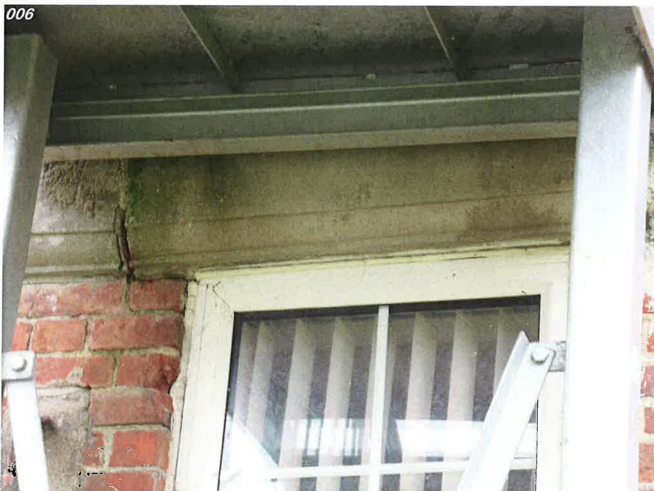
Displaced window head lintol
