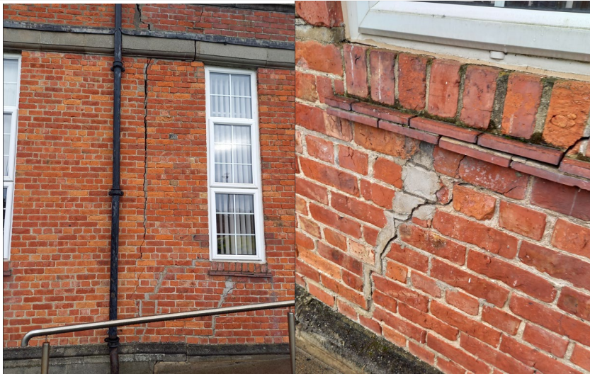
Above: exterior cracks on wall
