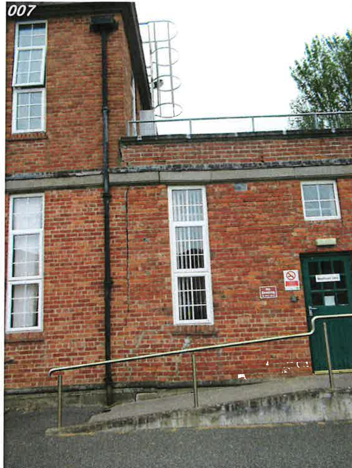
View of structural cracking along front of building
