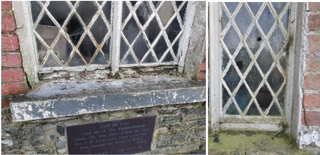
Decayed bottom rail
