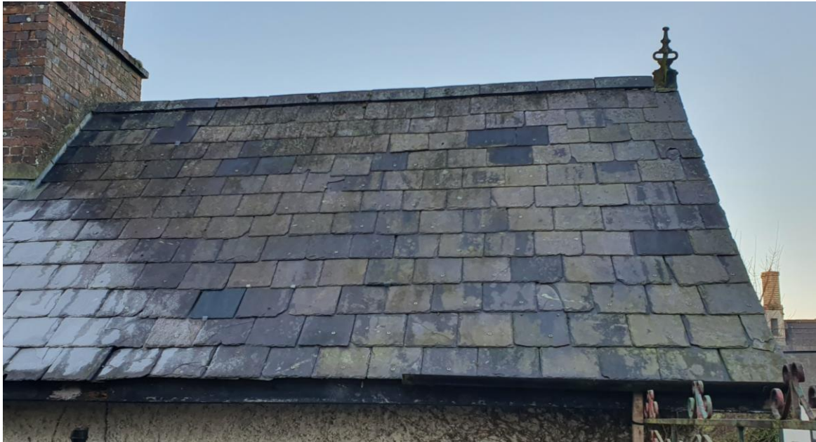
Southern pitch – cracked & slipped slates, numerous drilled holes, tings, portion of cast iron gutter
