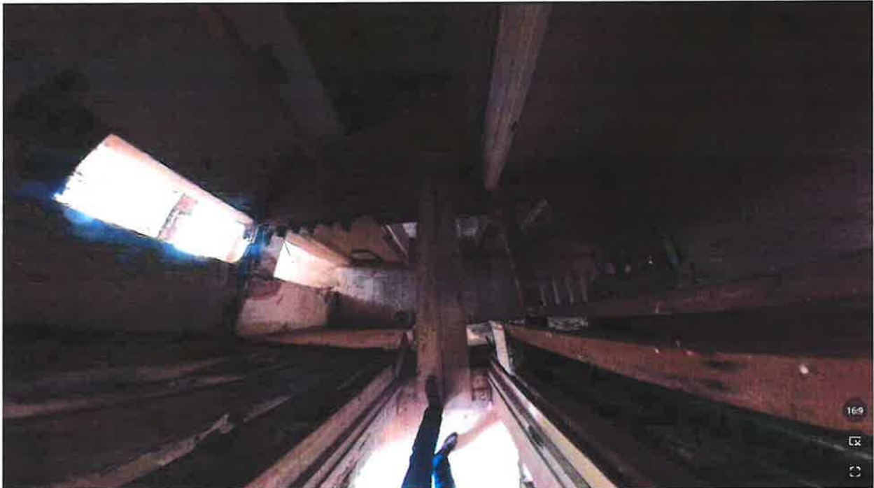
Figure 15 - Badly rotted floor structure
