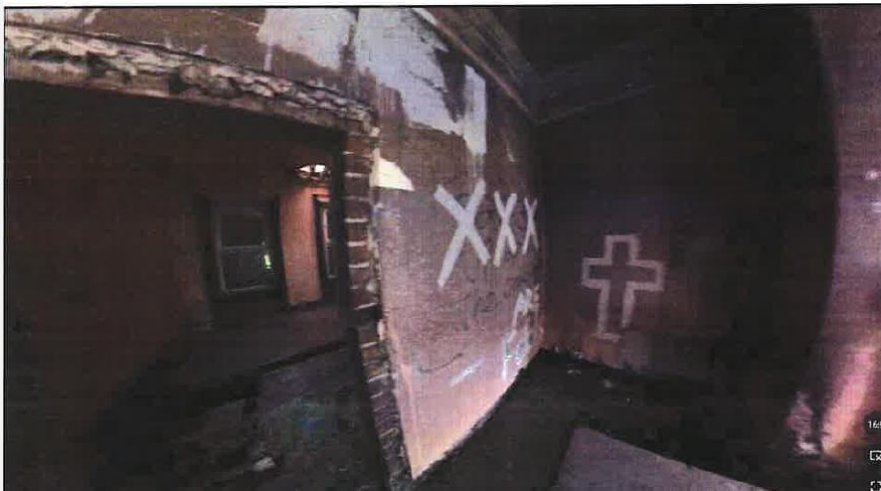
Fire damage and graffiti
