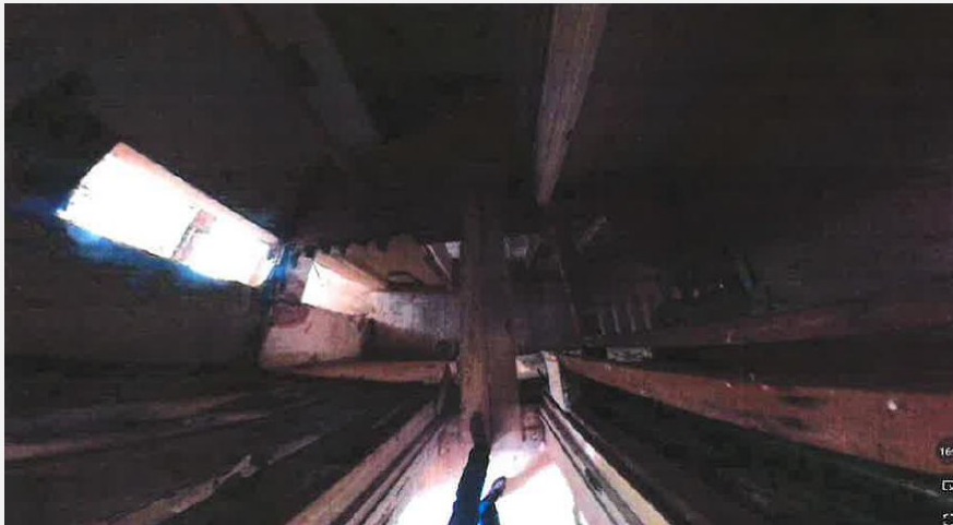
Badly rotted floor structure
