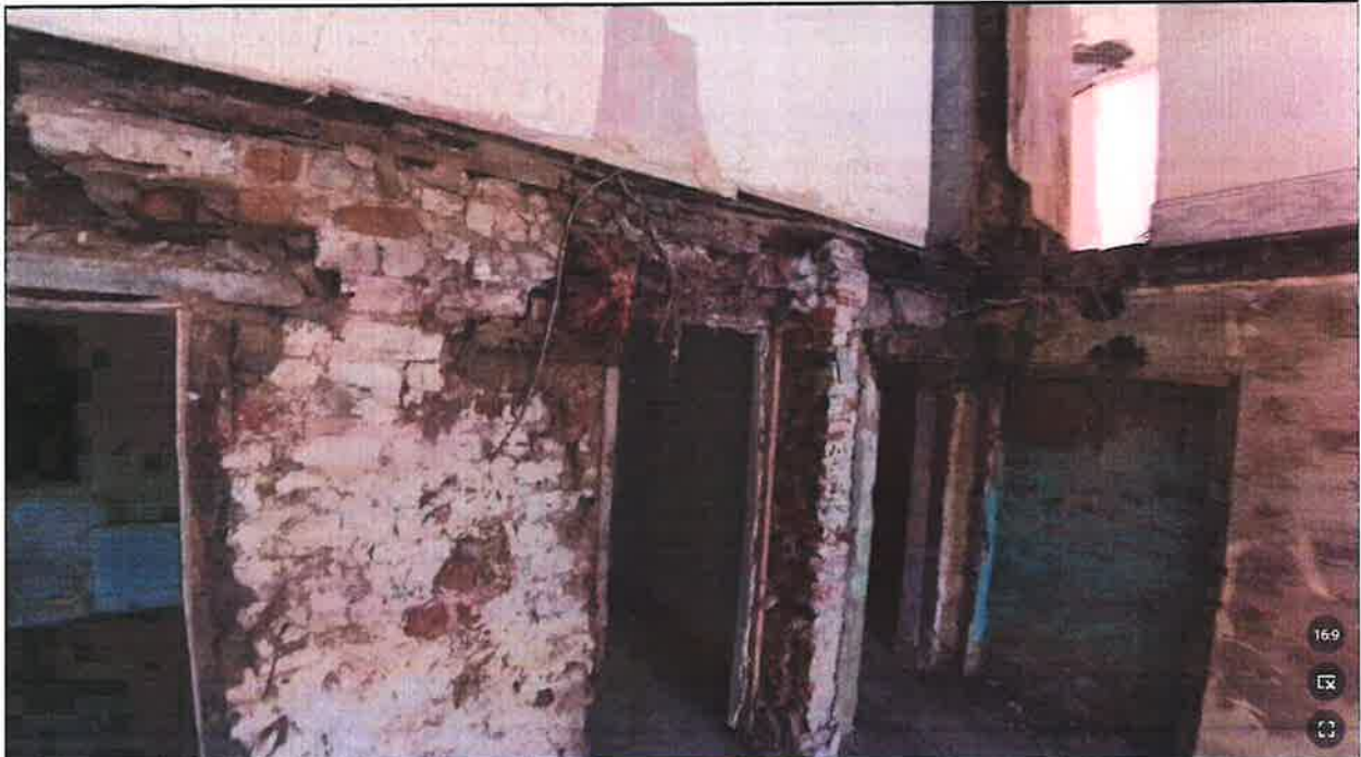
Figure 7 - Damaged finishes, removed floors
