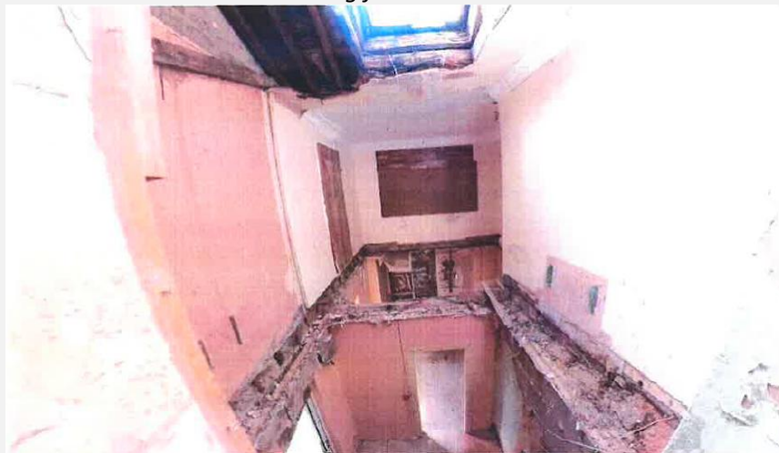
Missing floor structure
