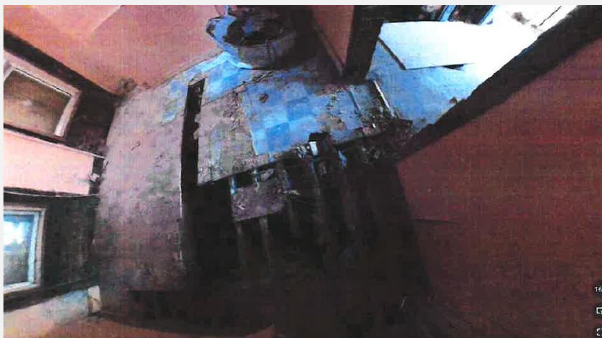
Badly rotted floor structure
