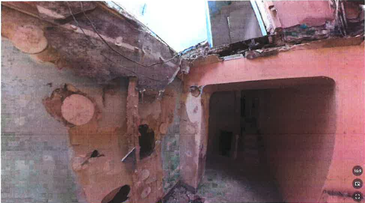
Figure 11 - Missing floor structure
