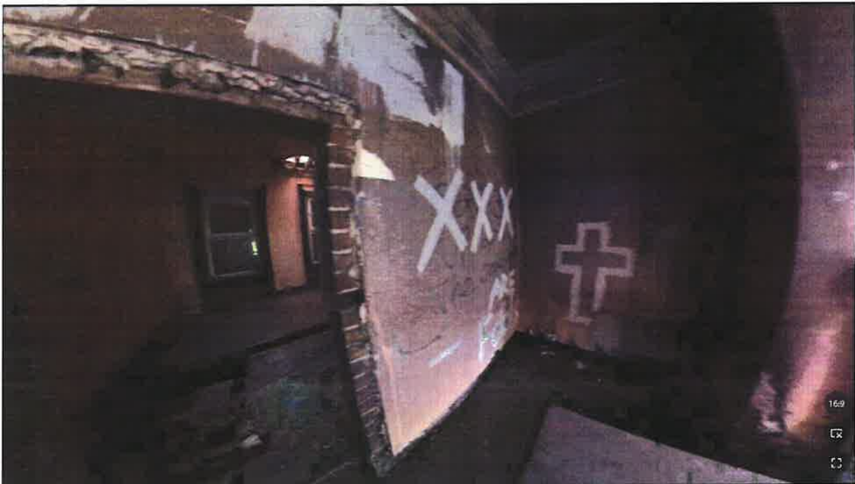
Figure 9 - Fire damage and graffiti
