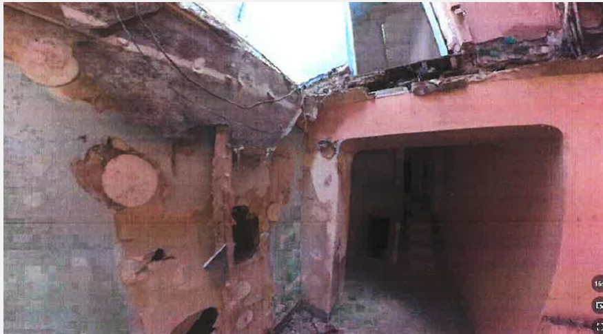
Missing floor structure
