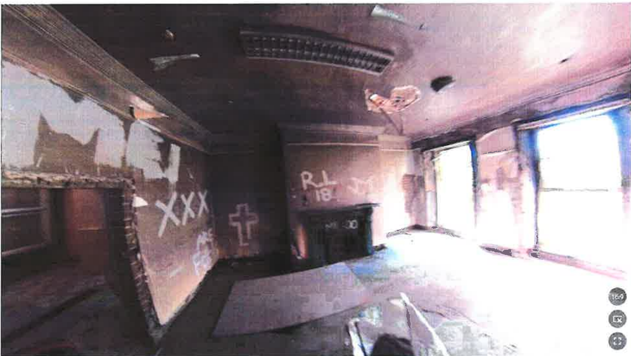
Figure 10 - Fire damage (walls and floor)
