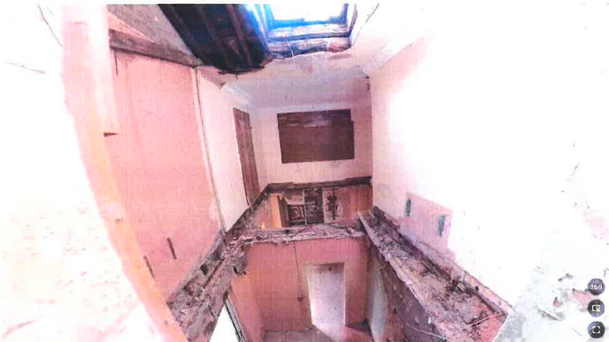
Figure 12 - Missing Floor Structure
