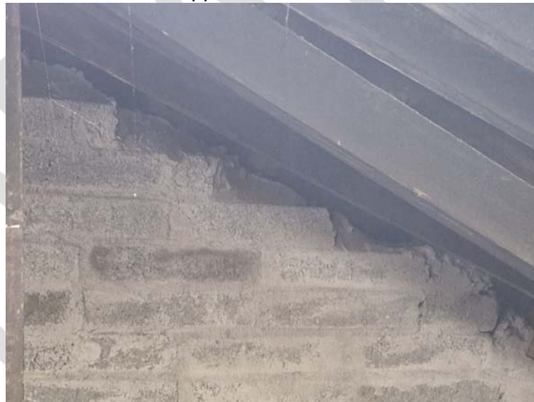
Photograph 2 – Adequate fire stopping to be provided
