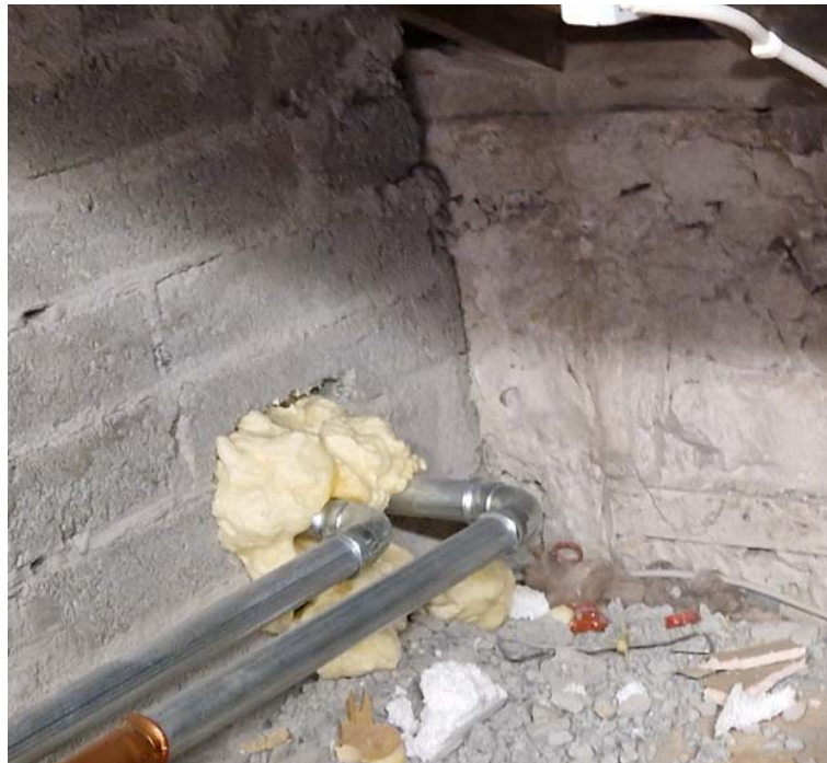
Photograph 6 – Fire stopping required
