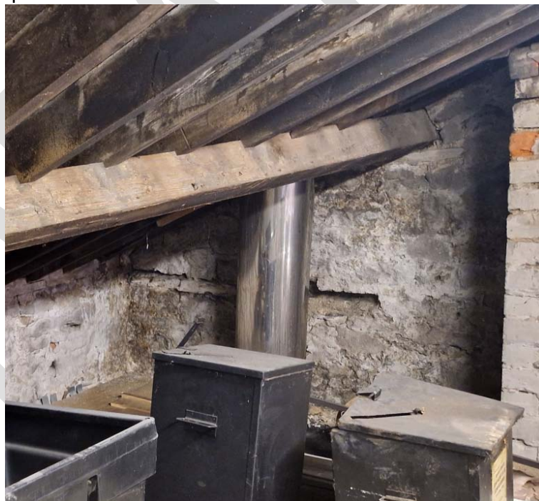
Photograph 7 – Fire stopping required
