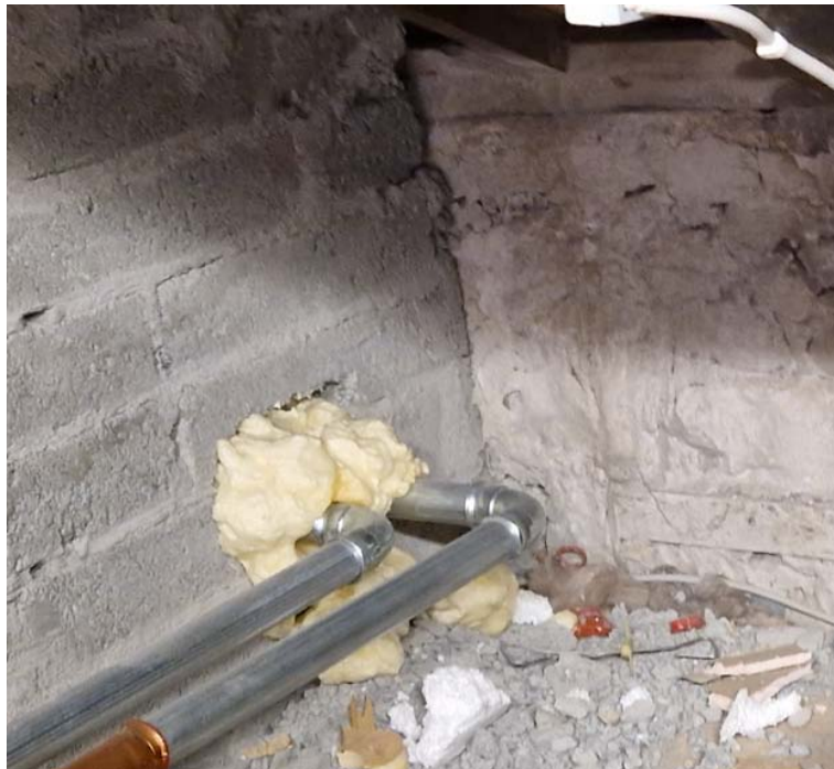
Photograph 6 – Fire stopping required
