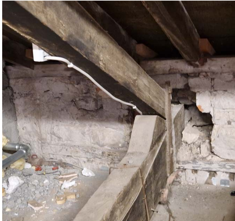
Photograph 8 – Section of wall to be rebuilt
