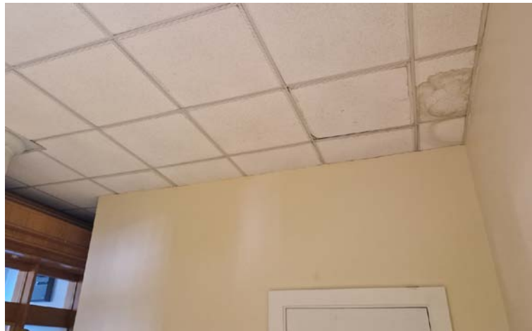
Photograph 21 – Water staining on ceiling tiles
