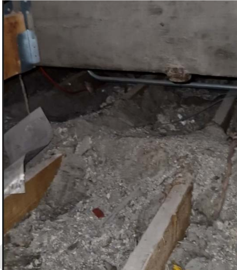
Photograph 18 – Debris on insulation
