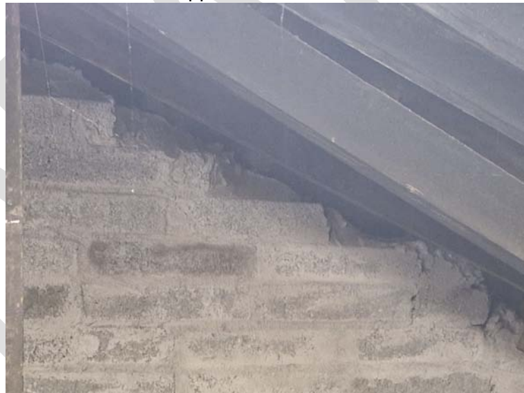
Photograph 2 – Adequate fire stopping to be provided
