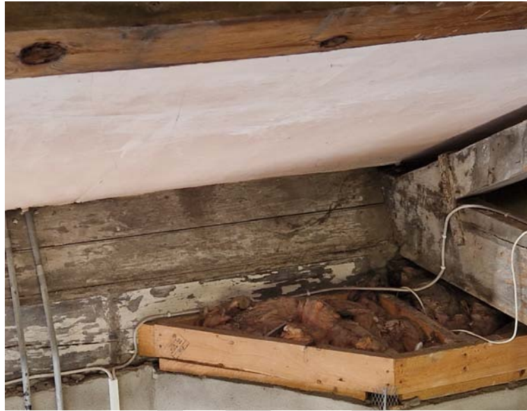
Photograph 5 – Lack of air gap between insulation and underside of roof
