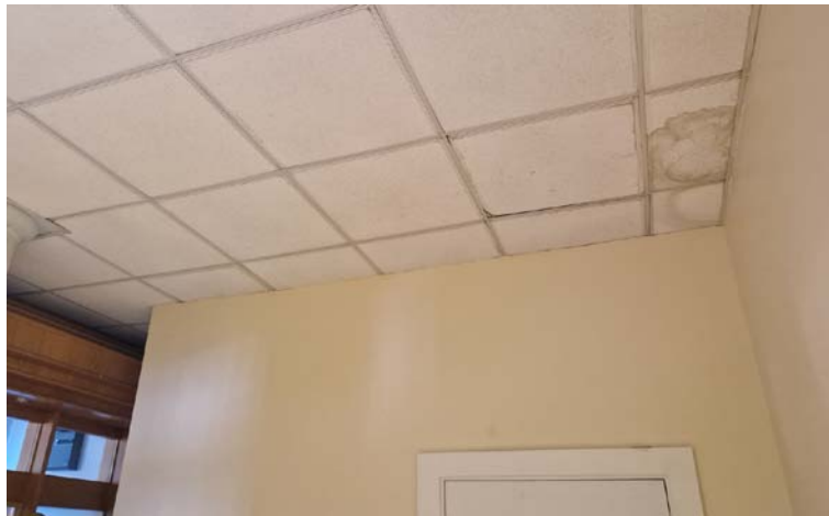
Photograph 21 – Water staining on ceiling tiles
