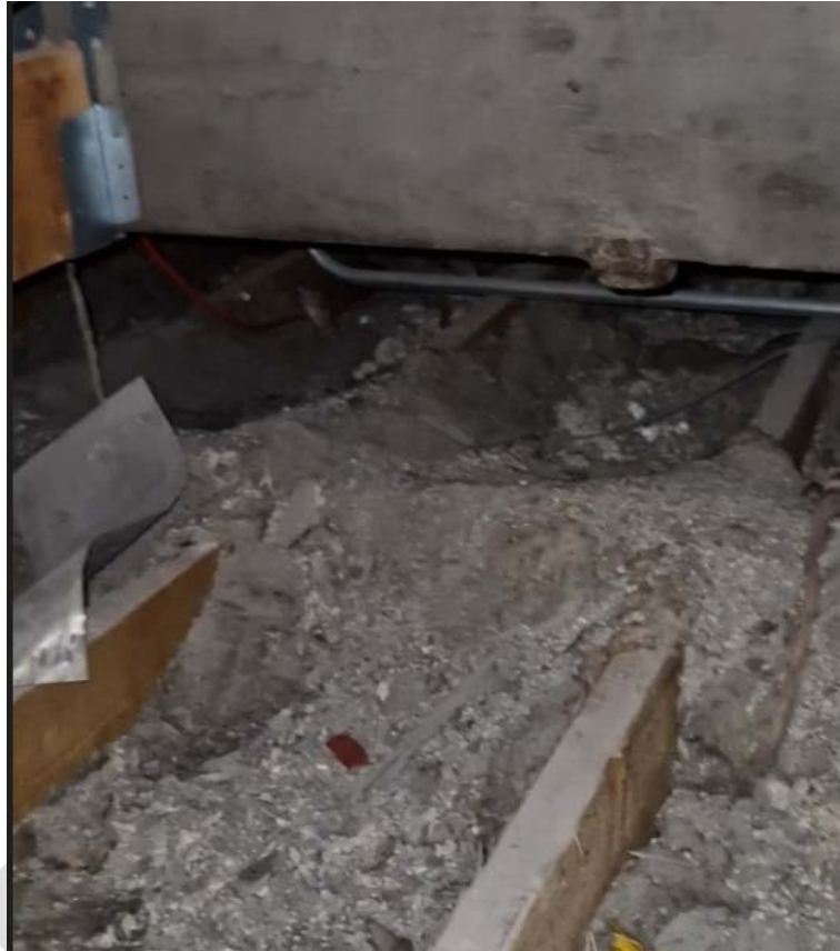
Photograph 18 – Debris on insulation
