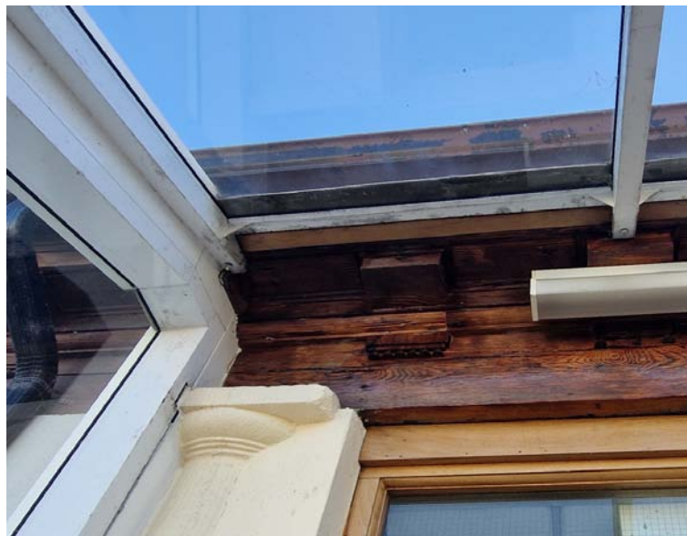
Photograph 23 – Water penetration at lean-to
