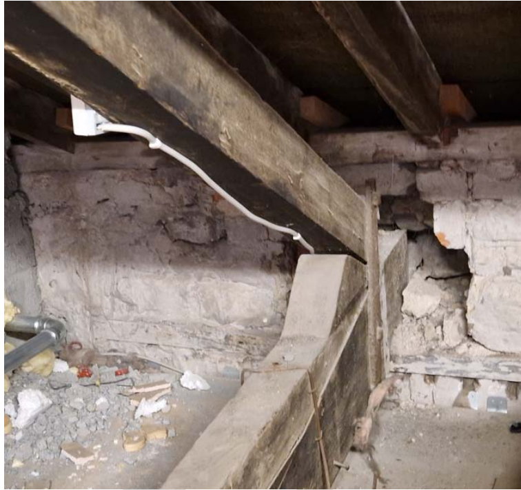
Photograph 8 – Section of wall to be rebuilt
