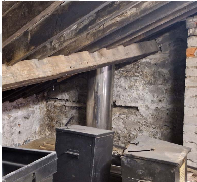
Photograph 7 – Fire stopping required
