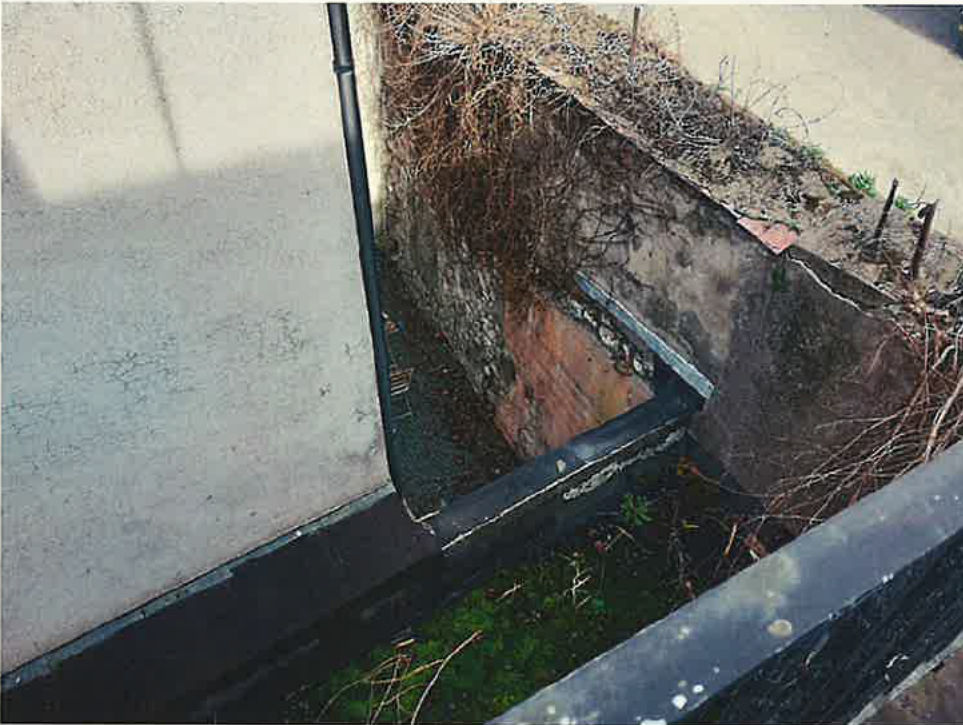
Photograph 3: Photograph taken from flat roof of part two-storey extension looking down onto the flat roof of the single storey extension. Applicant advised during site inspection that the extension is to extend to the end and be two-storey in height
