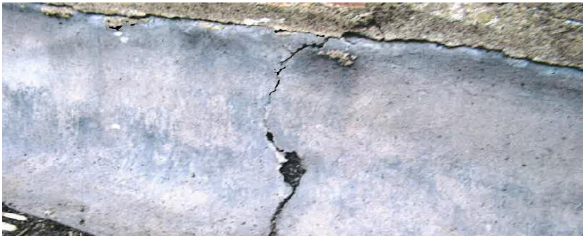
Damage to lead cavity trays.
