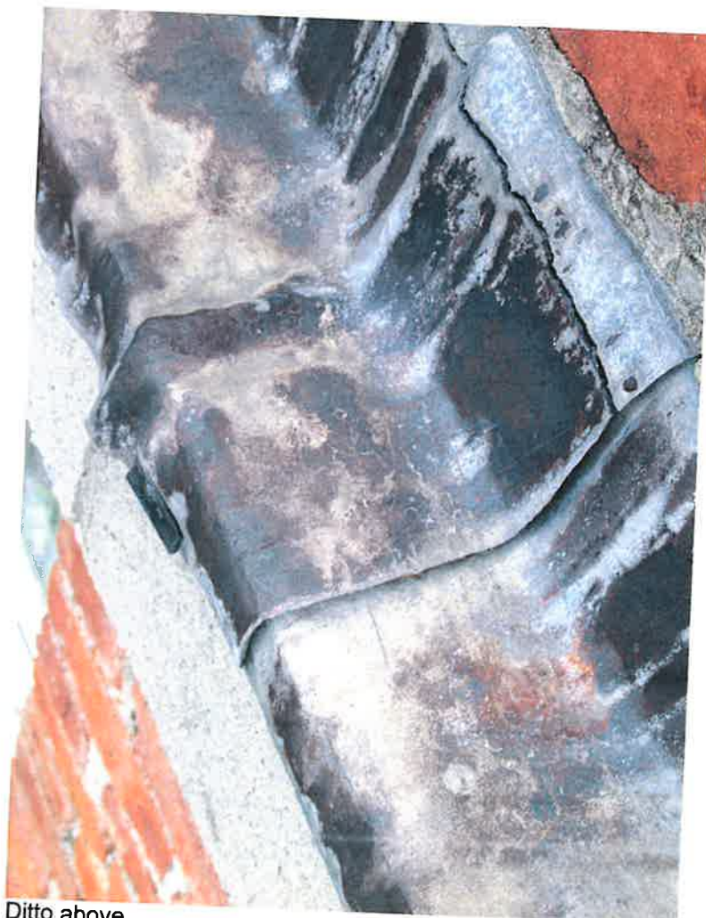
View of cracked and torn lead work
