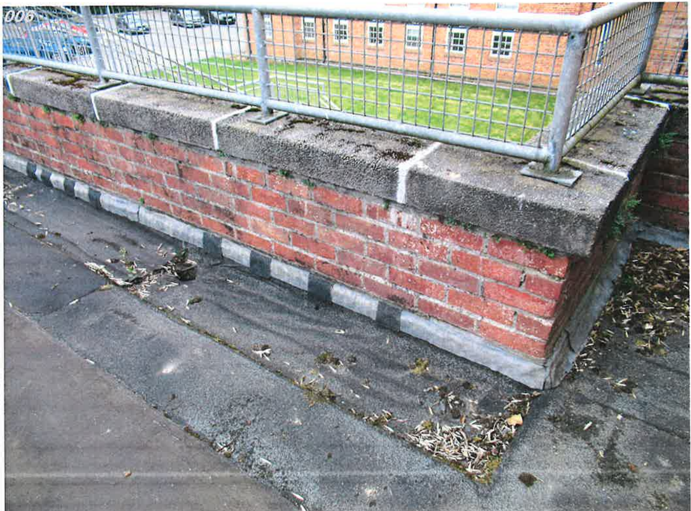
View of numerous patch repairs to lead cavity trays due to deterioration
