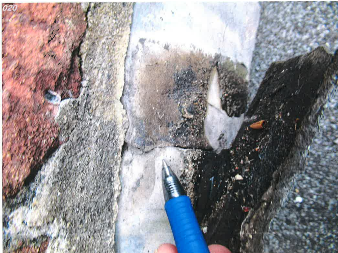
View of tears to lead work to flat roof
