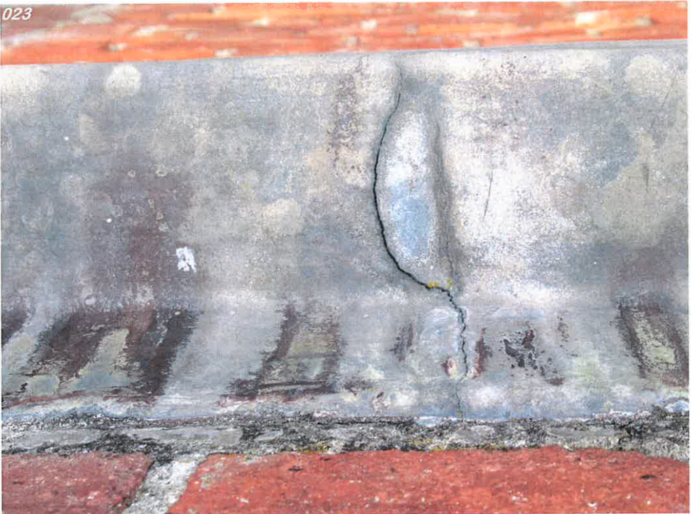
View of tears to lead work roof 2
