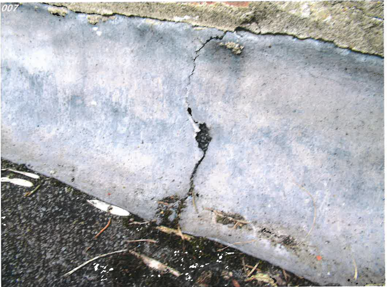
View of tear and cracks to lead cavity trays roof 3
