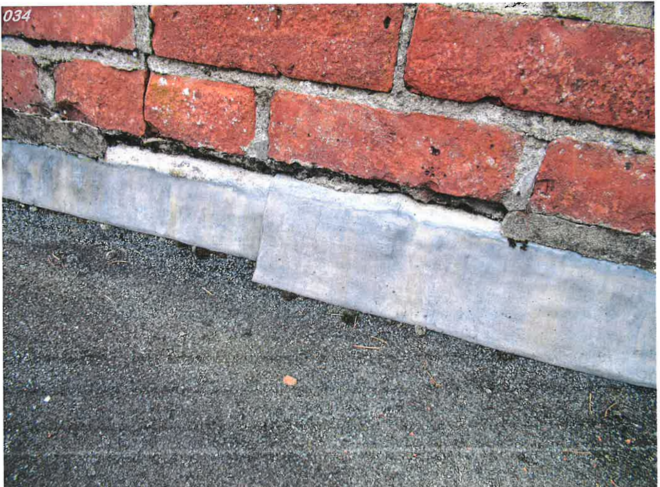
View of deterioration to parapet walls to be reconstructed
