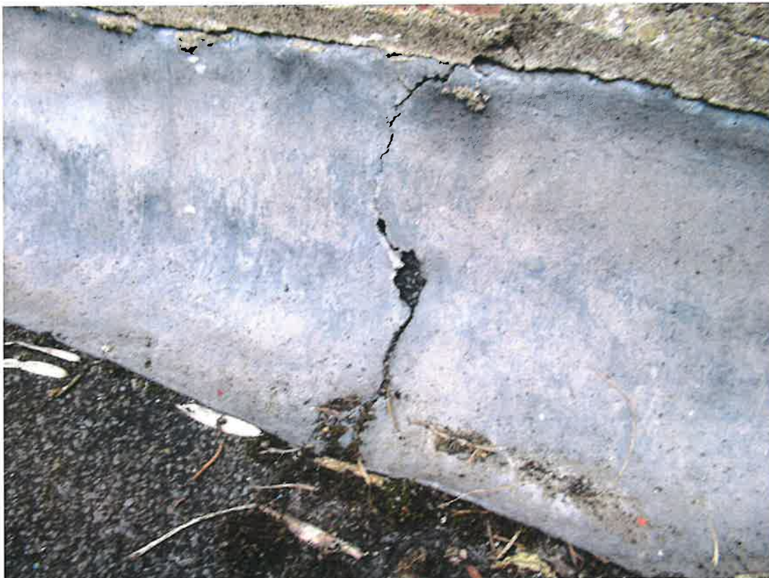
Image of cracked and torn lead cavity tray in parapet wall. Lead is 93 years old.
