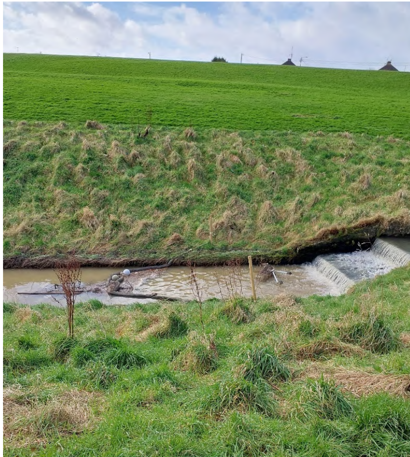
Plate 25. Ground photograph of the Glen stream (FW2) taken in April 2024 showing the floating boom, positioned downgradient of the stepped weirs, collecting debris before it enters the culvert. Note the grassy earth bank verge (BL2) along the edge of the stream.
