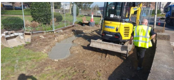
Dundalk World War I Memorial under construction at the Crescent, Dundalk, Co. Louth
