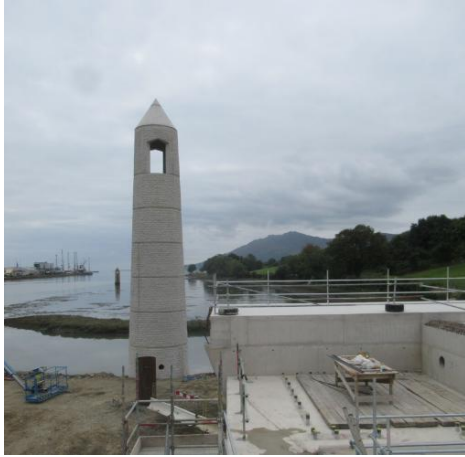
Navigation beacon tower
