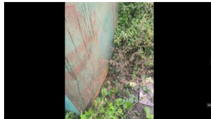
Sewage overflow from pumping station
