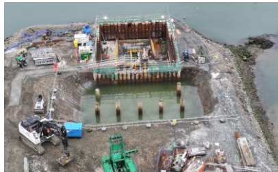
Aerial View of northern Bascule Chamber and commencement of the excavation for the Plant Room.
