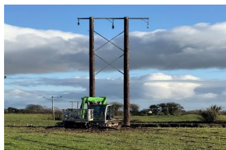
High Voltage ESB Network Diversion
