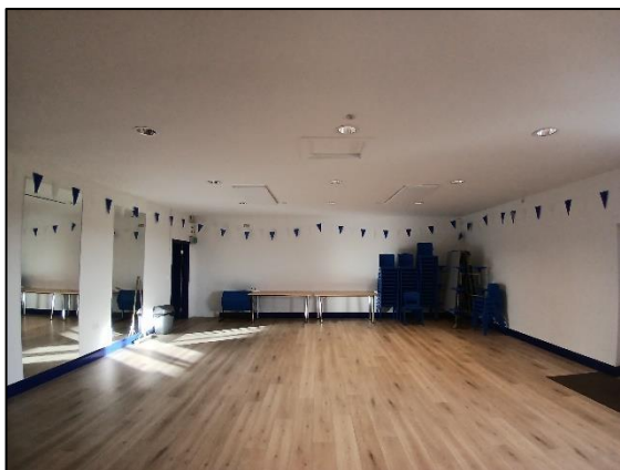
Photos from Naomh Mairtin GAA club who have recently installed infrared heating panels under the Community Climate Action Fund.
