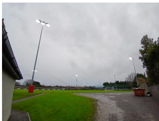
New LED lighting at Drogheda Town F.C
