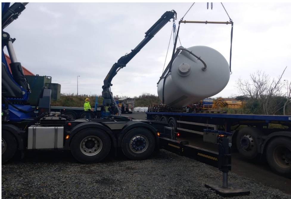
New salt silo at Faughart yard
