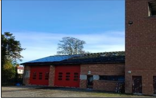
Photos Recently completed 39 x panel, 17.4 kWp array at Ardee Fire Station.
