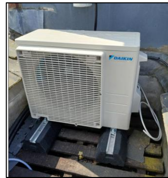
Photo: New Air Conditioning unit at County Hall (the stationary room).
