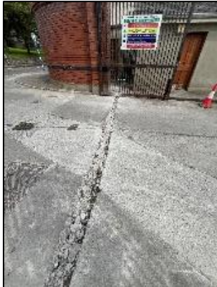
Photos: Removal of Old Barrier Equipment; New Safety Sensor and Access Control for Gate and Cutting of Tracks for Ducting
