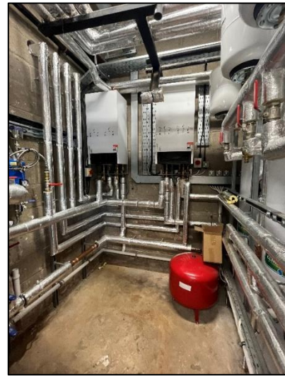
Photo: New Pipework at Dundalk Fire Station's Plantroom
