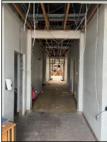
Photos: Demolition and 'Opening-up' Works at the Cornmarket Building at Fair Street, Drogheda
