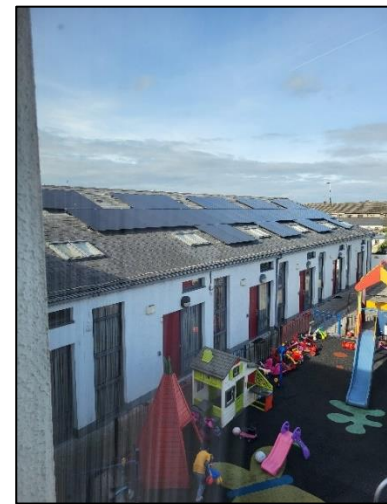
Solar panels that have recently been installed at the Drogheda Women and Children's Refuge.
