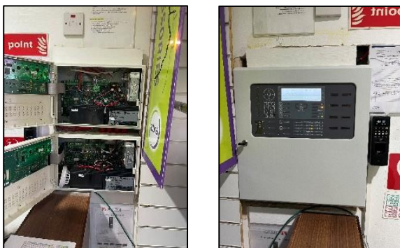
Photos: The old & new Fire Alarm Panels at Drogheda Leisure Centre.
