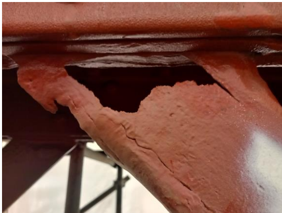
Typical Loss of cross section at Lattice Members
