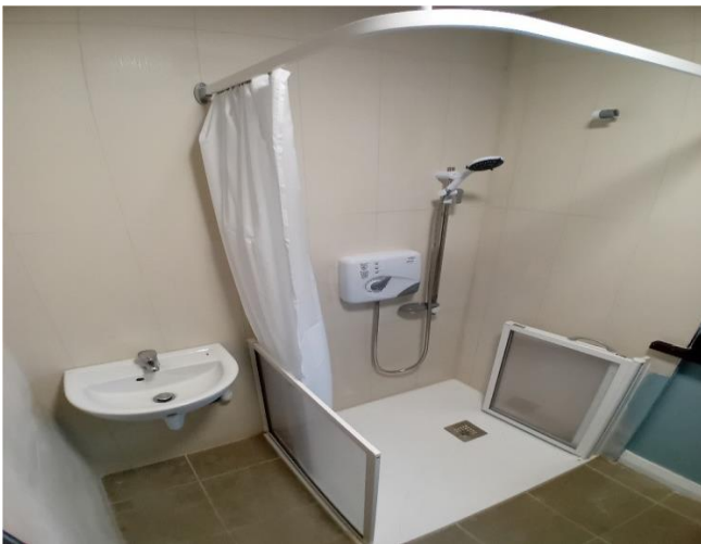
Level Access Shower completed in Dundalk during November part-funded by a HAG
