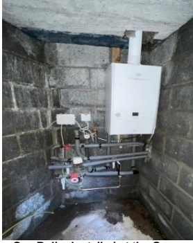
New 30kW condensing Gas Boiler installed at the Governors House, Millmount, Drogheda
