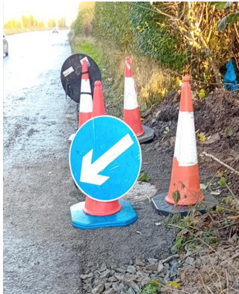
Drainage on the N33
