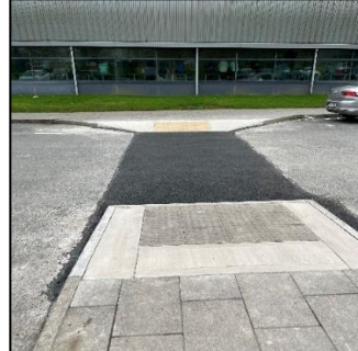
Cleaning and adjustment of tactile paving for the new crossing point at Drogheda Aura Leisure Centre
