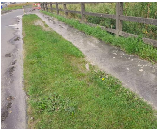
Blocked sewer Drogheda which discharge to the Boyne
