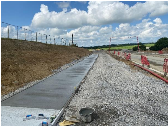
Ch.750 - 900m Concrete pour to footpath west of bus bay, southern side of road
