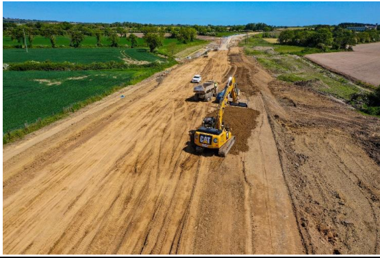
Ch.0 - 200m east of Rosehall roundabout installing/compacting selected material underneath capping layer
