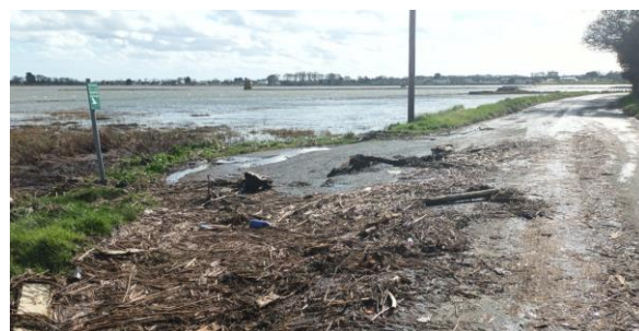
Debris washed onto the R167 from High Spring Tides that flooded road
