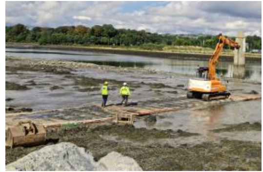
Mud Mats installation to allow access to the proposed works Roost Site Works
