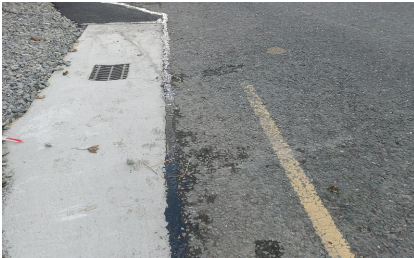
New Drainage installed at the junction of the R132 with the LS-6274-0 Gallstown Road
