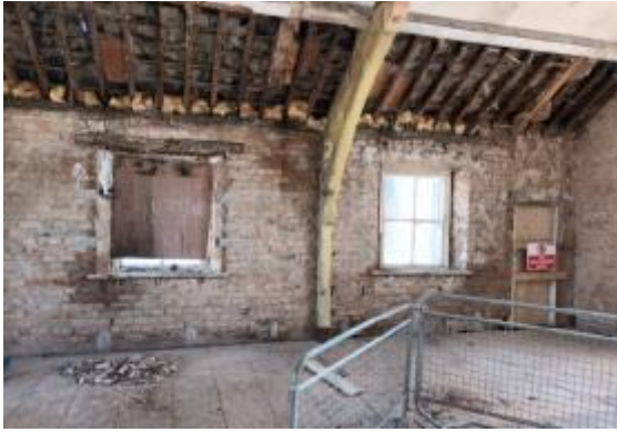
Strip of plaster at window reveals and heads revealing extent of dry rot
