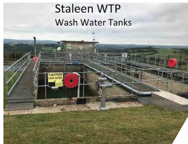
Staleen Water Treatment Plant
